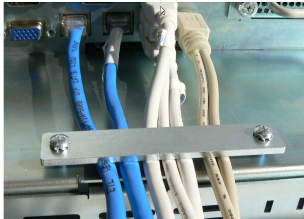
Cable Securing Bar Installed
